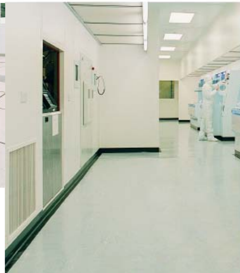
POLYFLOR SD - CLEAN ROOM
